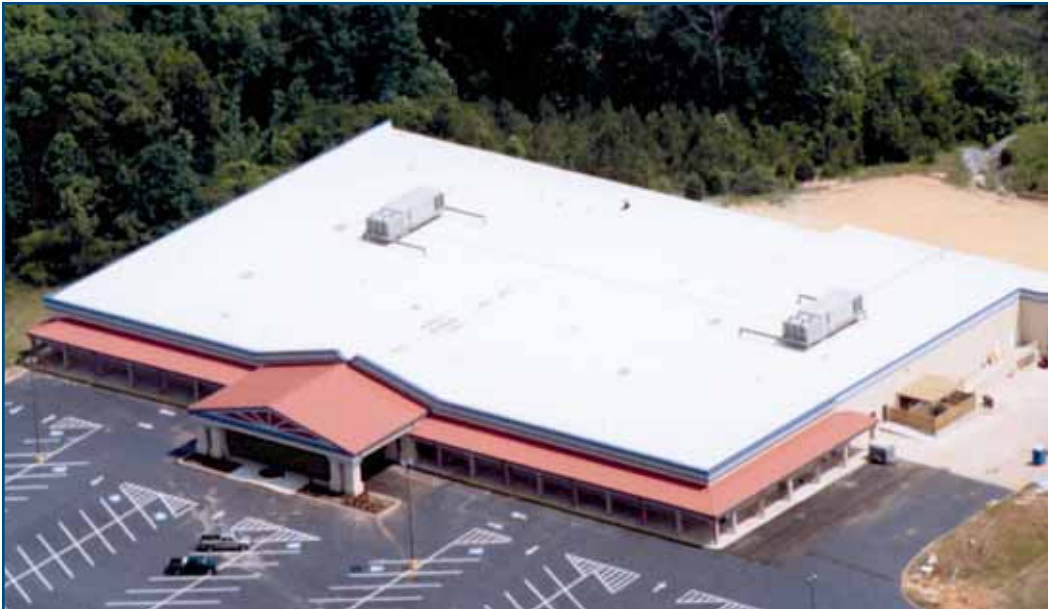
Photo 4 – Cool roofing systems are especially effective on low-rise buildings with large roof areas. Potential energy savings during the hot Mississippi summer months helped convince the Grenada Medical Complex in Grenada, Mississippi to install a recyclable, high-performance thermoplastic cool roofing system covering 69,474 square feet. (Photo courtesy of Duro-Last Roofing, Inc.)
